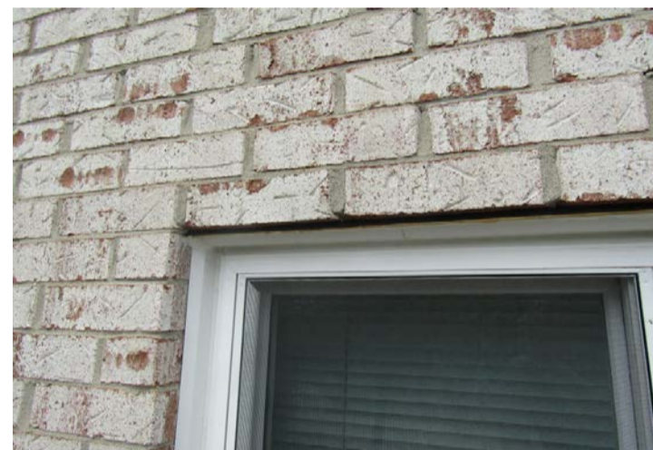
rust at lintel
