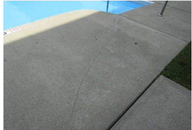
minor crack in deck concrete
