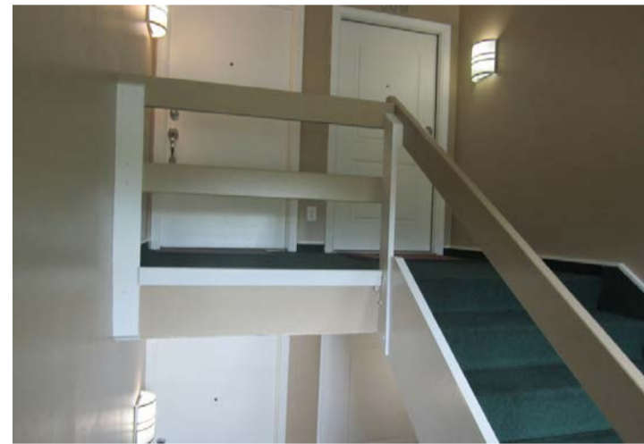
missing balusters at railing
