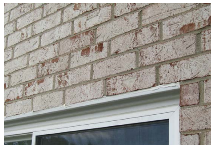
cladding and caulk inappropriately installed over lintel
