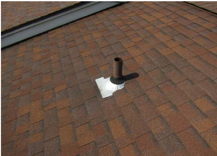
unsecured flashing - semiannual inspections to address these conditions
