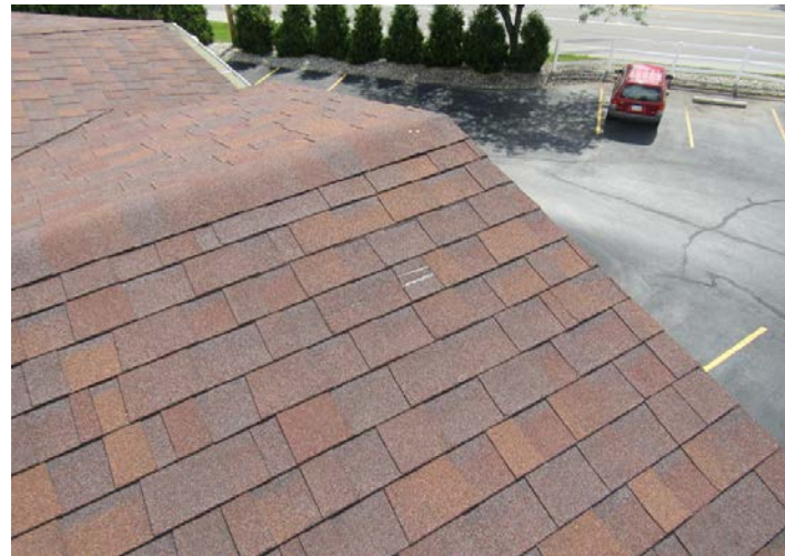
damaged shingles and fiberglass exposure
