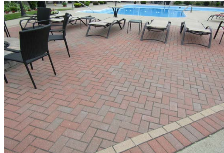
pavers at pool deck
