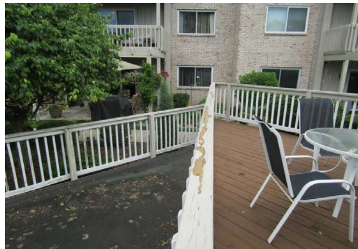
peeling paint at railing
