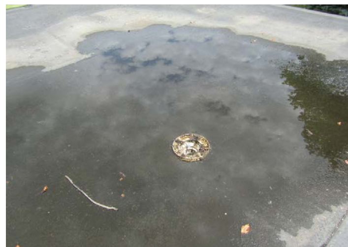
missing drain screen
