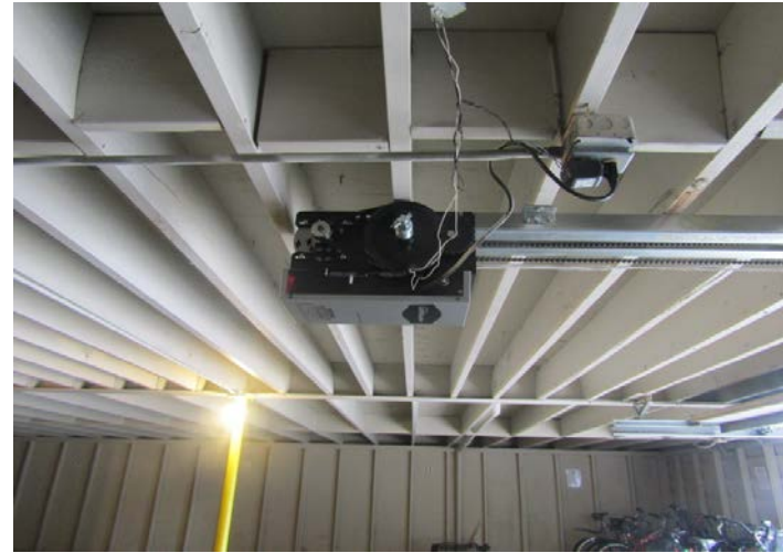
LiftMaster door operator
