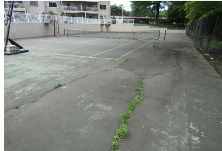
cracks in pavement
