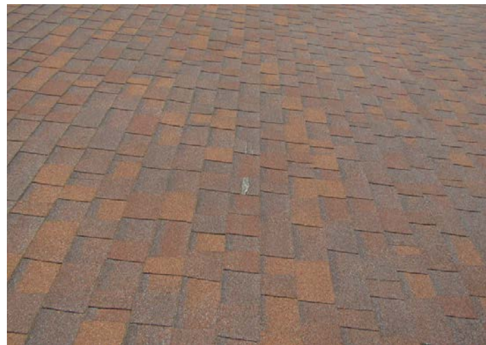
damaged shingles and fiberglass exposure
