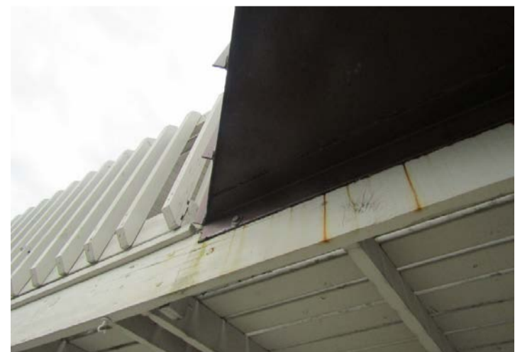
rust at staircase
