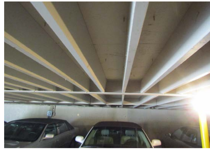
Painted surfaces in garage
