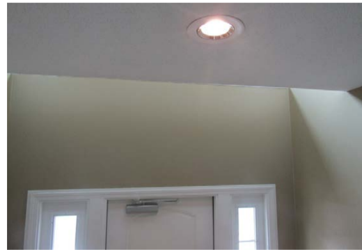
light operating during daylight
