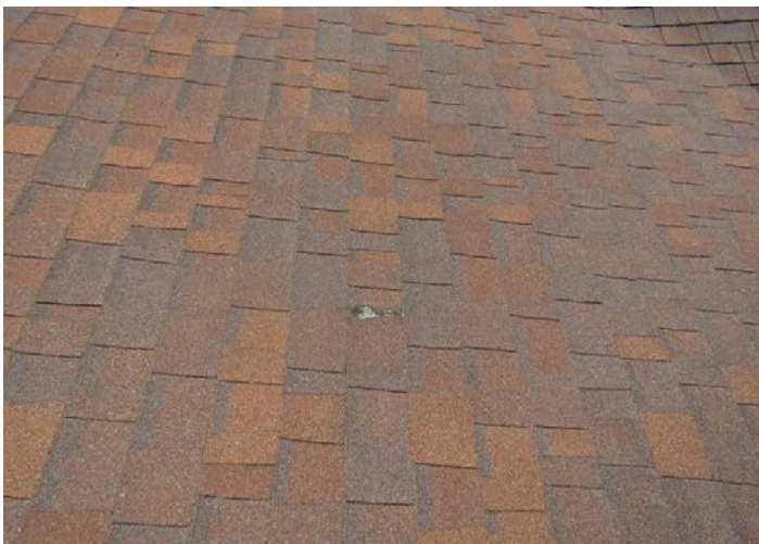
damaged shingles and fiberglass exposure
