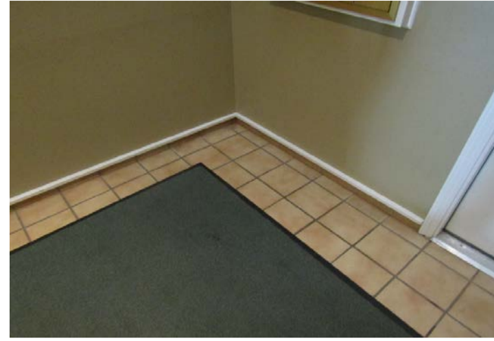
8 inch by 8 inch tile typical of the stairs with tile transition at floor to wall
