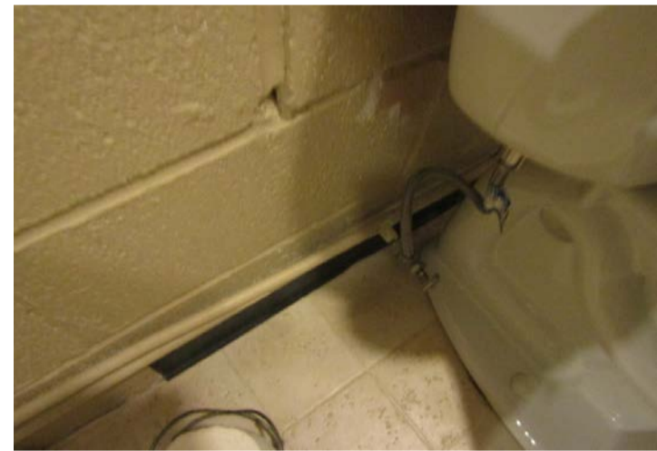
cold water supply pipe
