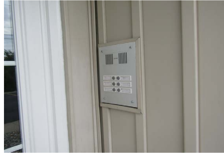
Aiphone intercom system panel
