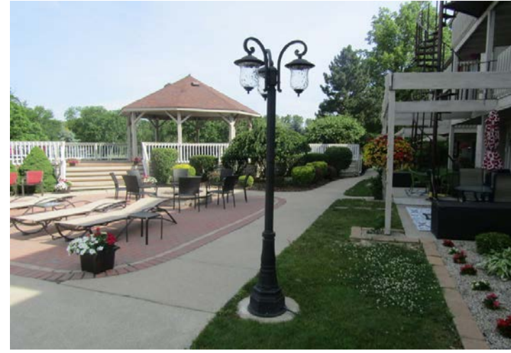
metal light pole with metal light fixture
