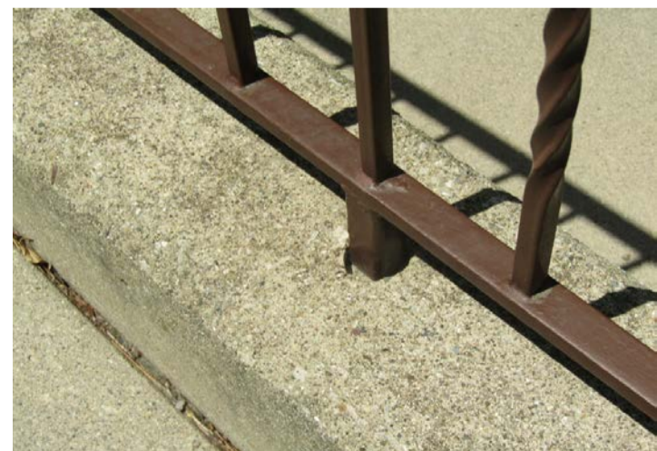
void at railing mount
