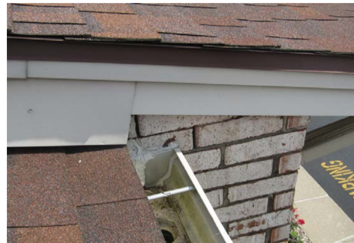
worn mortar joints
