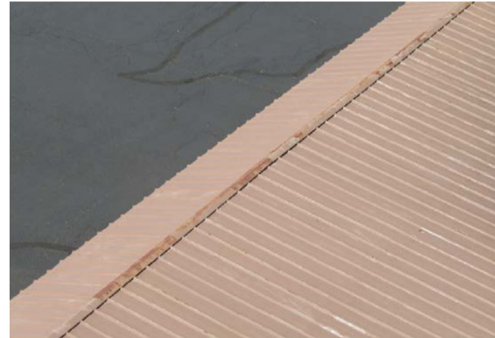
rust at metal
