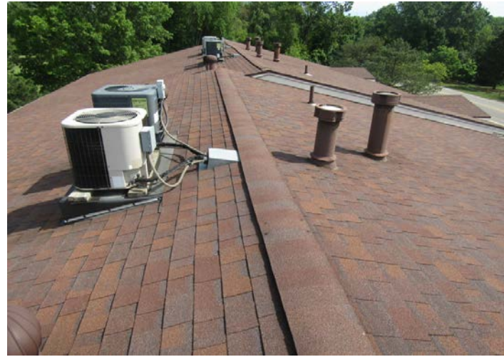
ridge vent without wind baffles
