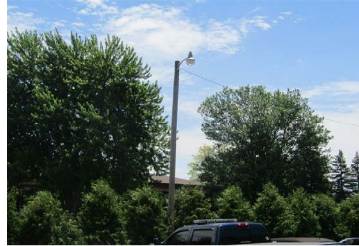
wood light pole with metal light fixture
