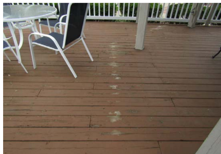
worn paint at deck
