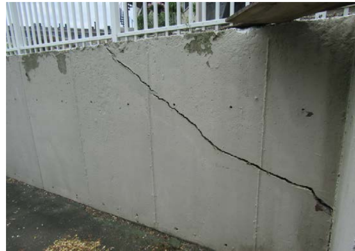
crack in concrete
