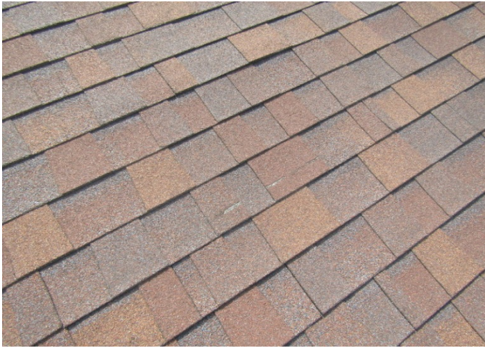
damaged shingles and fiberglass exposure
