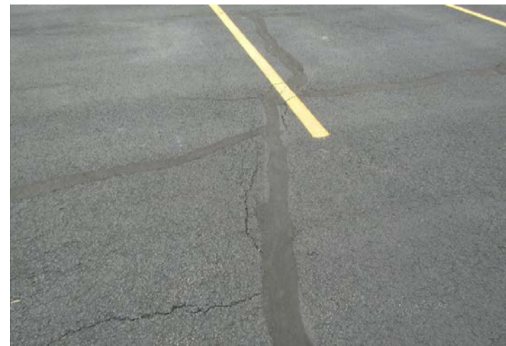
repaired and unrepaired cracks
