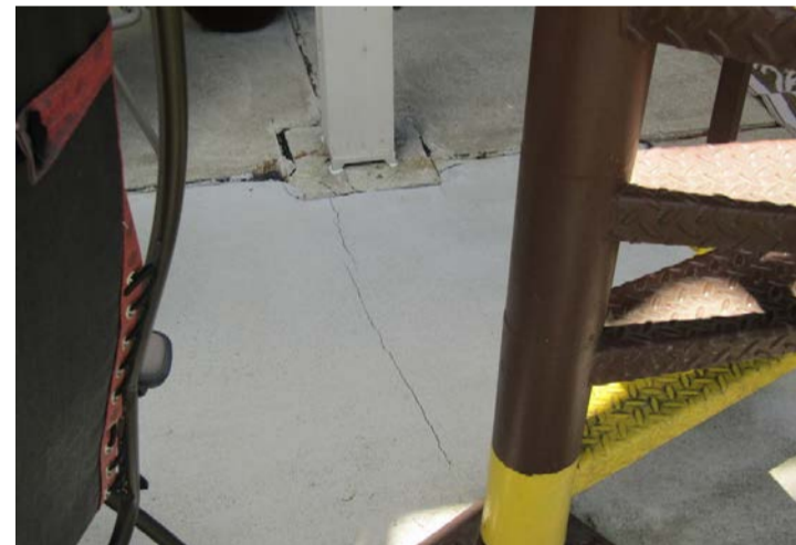
minor crack - no action necessary
