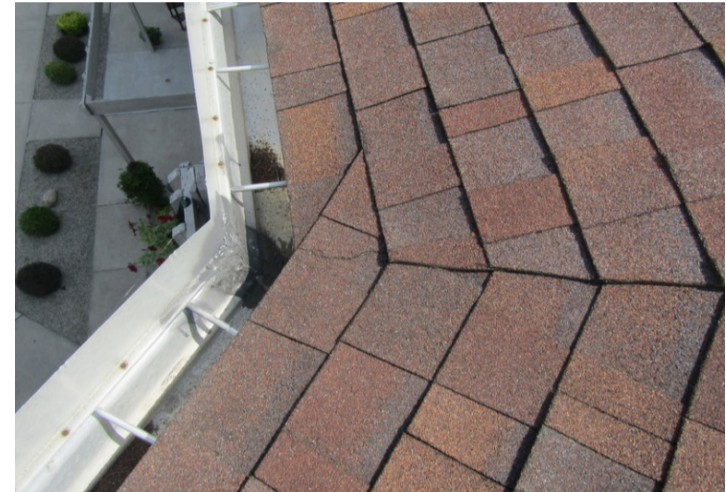
repaired gutter leak
