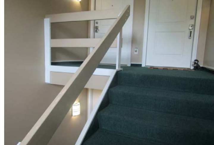
missing balusters at railing
